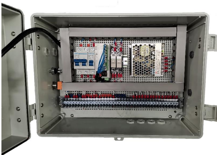
Figure 2. Wiring terminal and power circuit breakers
